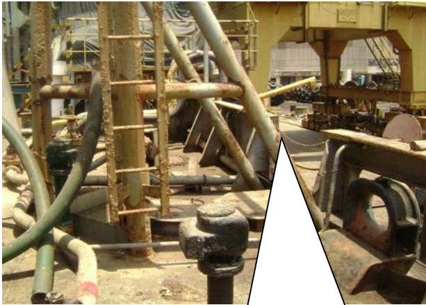
Existing Structure: Excessive corrosion & inadequate strength for New Boom
